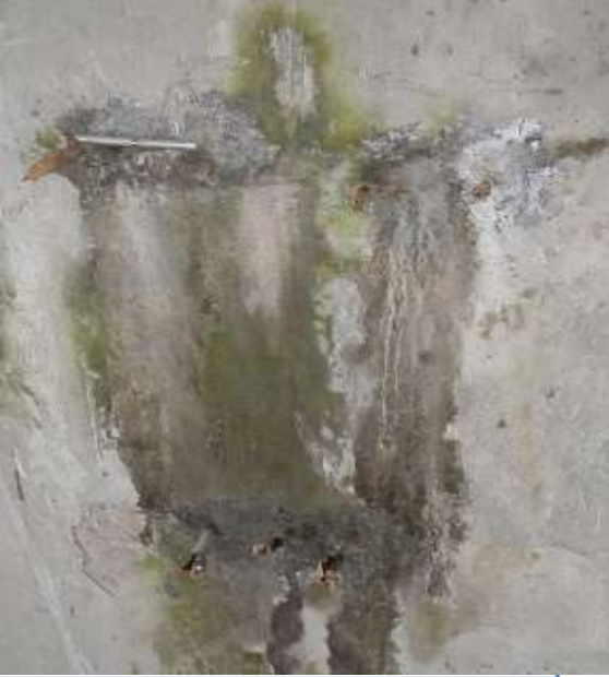
spot seepage on the wall W2
