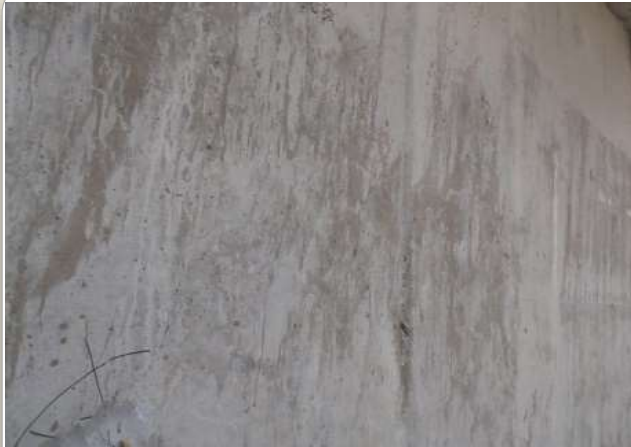
surface area seepage on the wall W1
