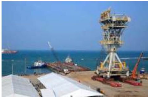
EPC-3 Offshore Pipeline, Mooring Tower and Support Structure
